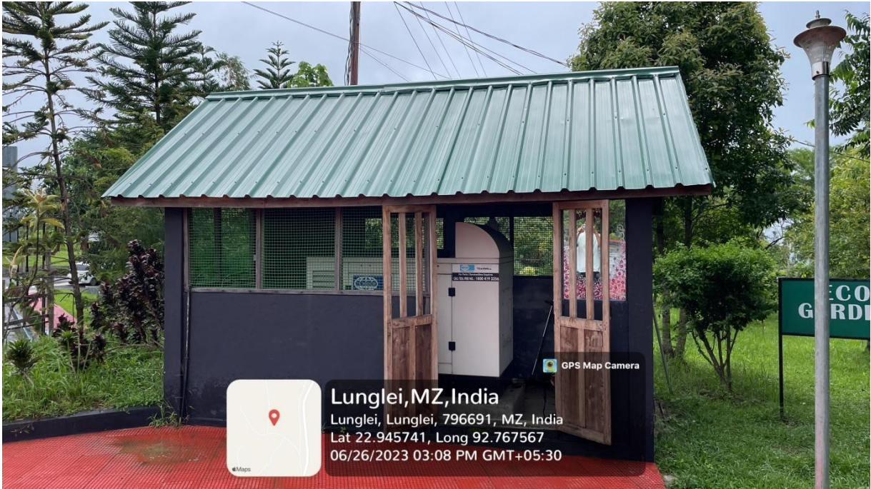
Pic: 25 KVA Diesel Generator
