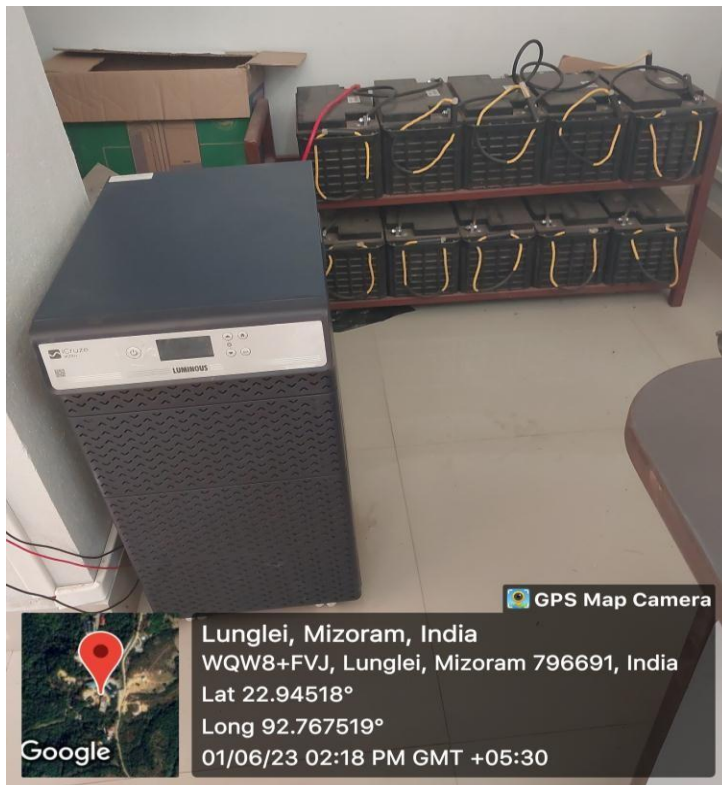
Pic: 10 KVA UPS with Battery at IT CENTER
